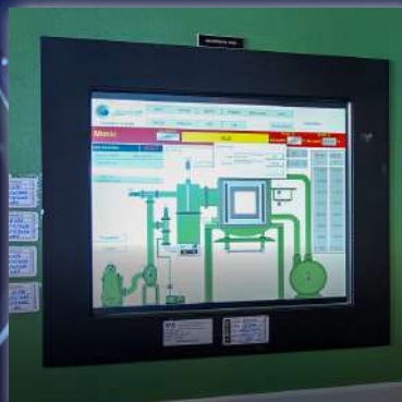
HEAT Treatment Shop
